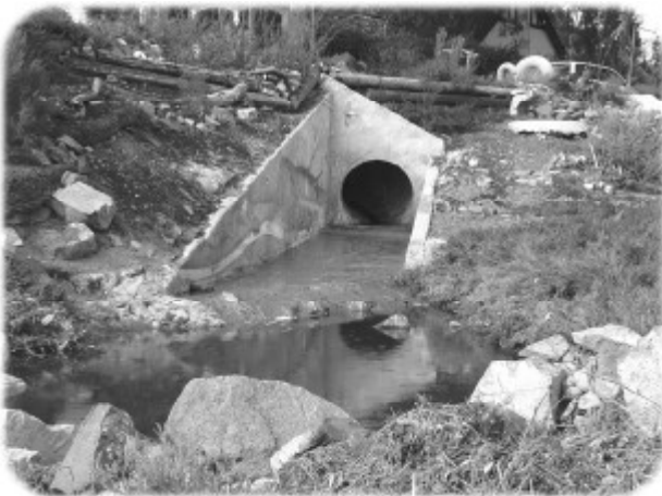
A storm drain outlet which flows unfiltered directly into a local stream.
