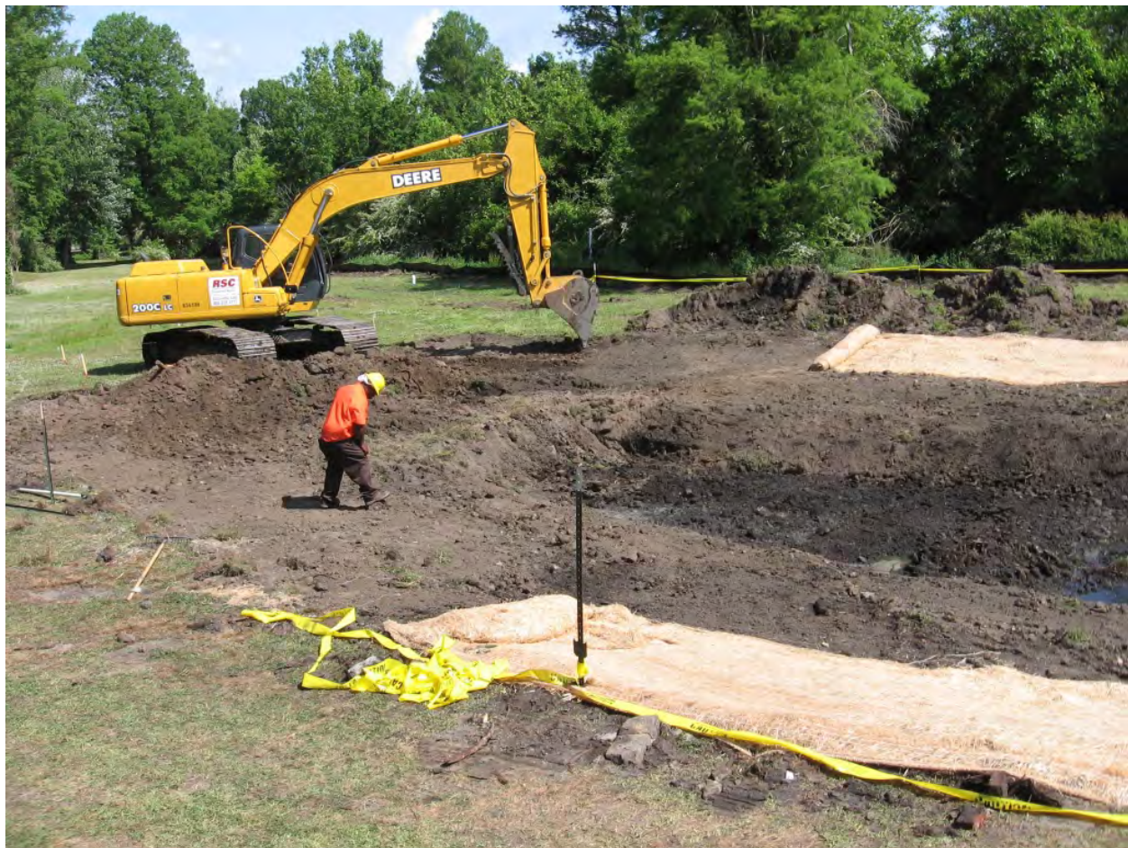
Figure 4-4. Heavy equipment (especially wheeled equipment) should be operated outside the excavated area to prevent compaction.
