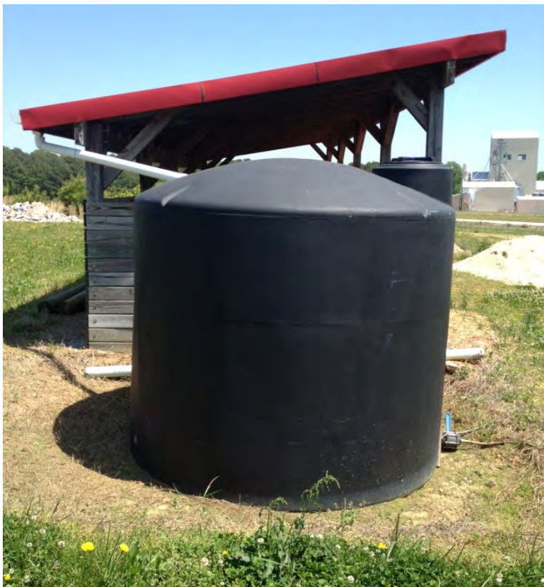
Figure 3-39. Typical plastic cistern.
