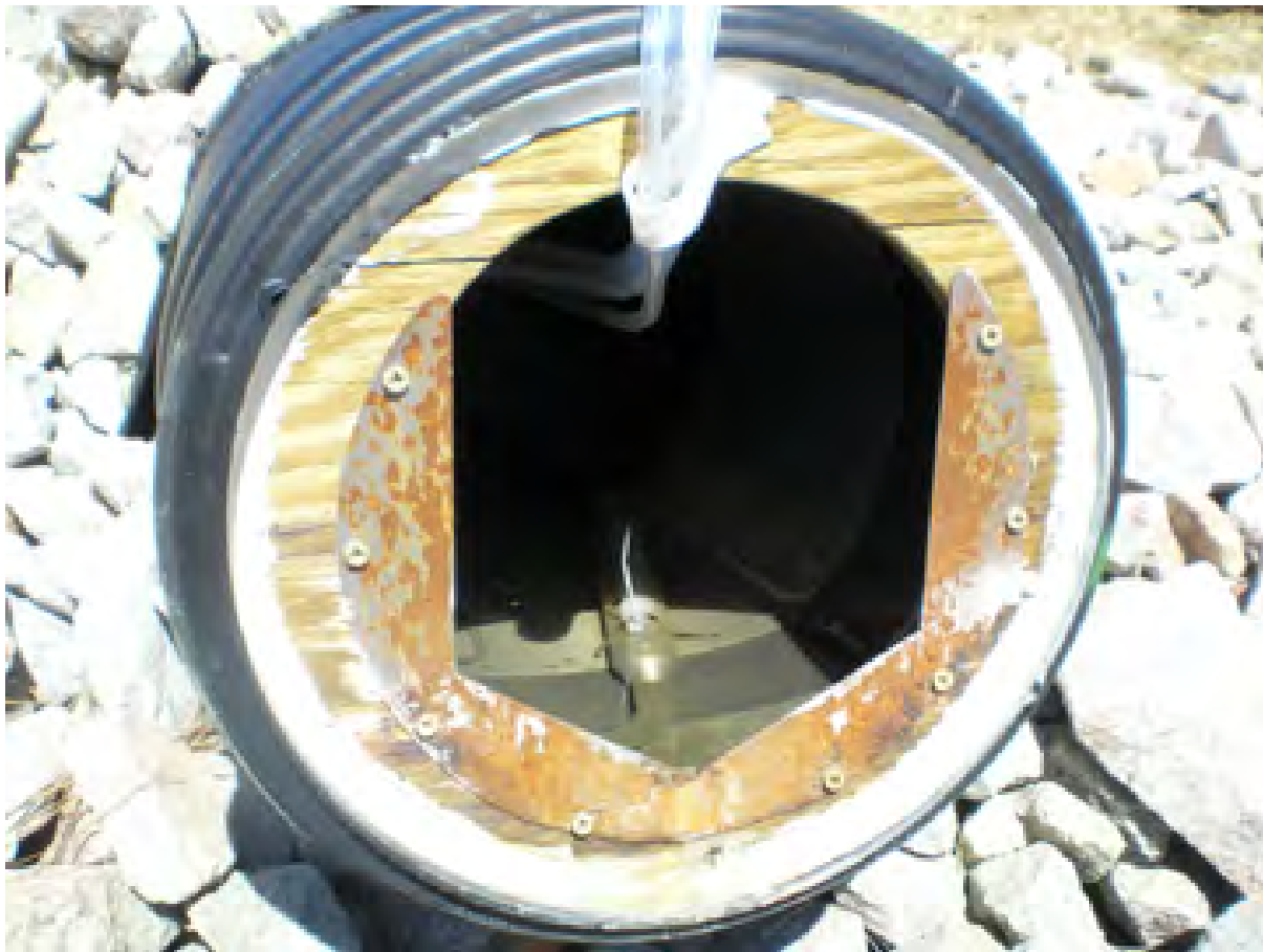
Figure 4-12. Inflow pipe to a bioretention area equipped with compound weir and bubbler for flow measurement. Water quality sampling tube and strainer are visible inside pipe.
