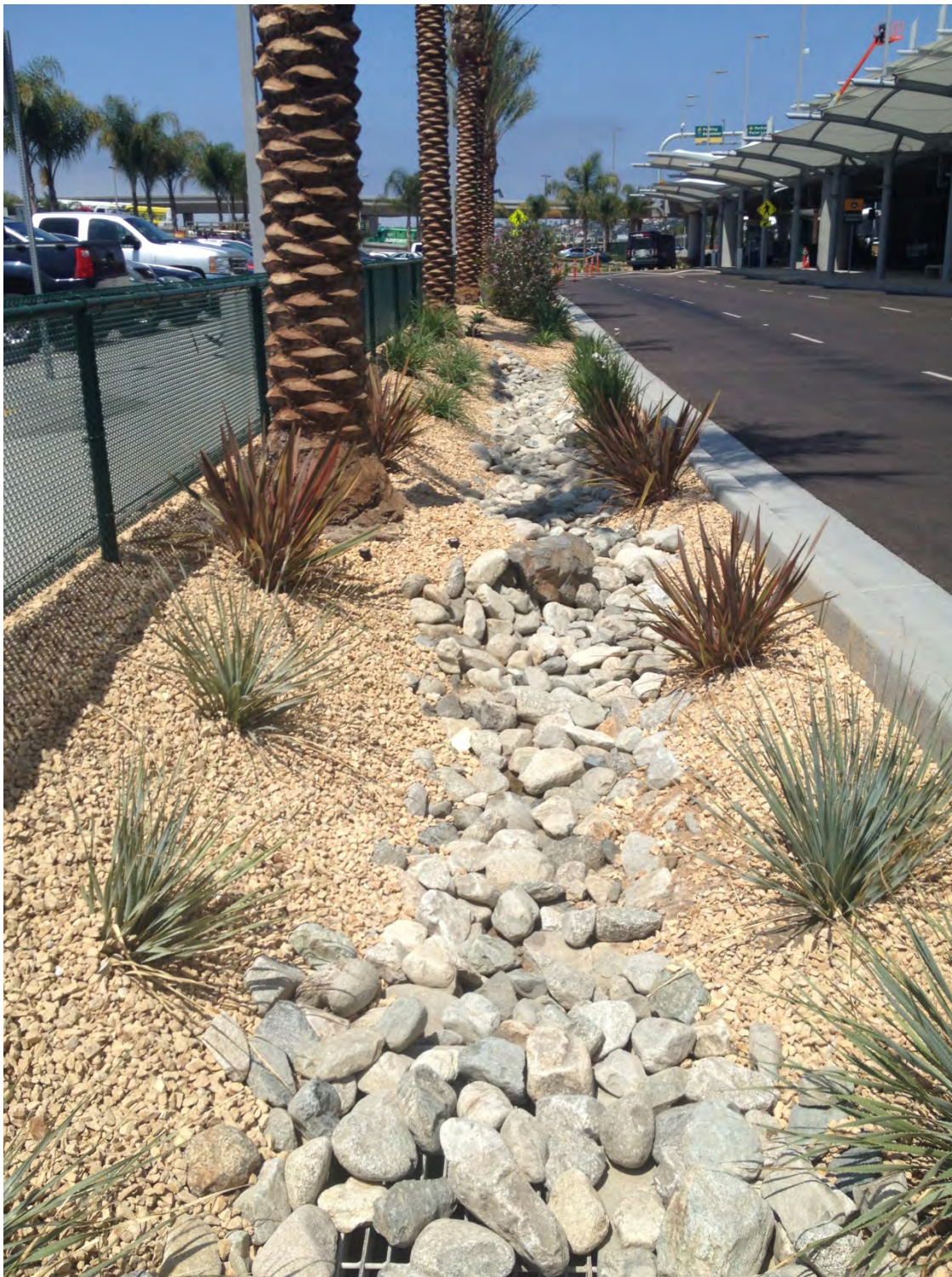
Figure 4-23. Cobble and gravel stabilize the surface of the rock infiltration swale and prevent scour of underlying soil media. The outlet structure in the foreground is elevated 2" above the bed of the rock infiltration swale to ensure that the design storm flow is retained and filtered through the media.
