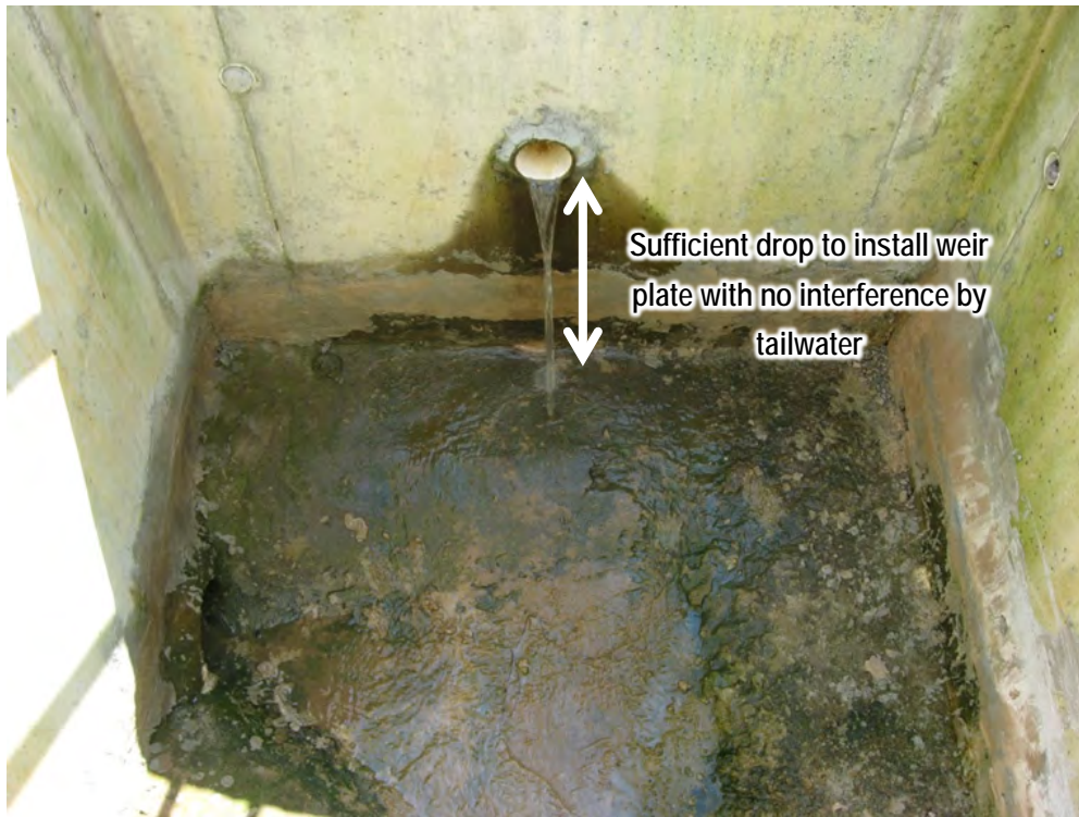
Figure 4-16. Example of a bioretention underdrain outlet with sufficient drop to install a flow monitoring weir without encountering tailwater.
