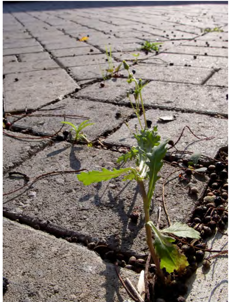
Figure 4-9. Plant growth, debris buildup, and puddles indicate that permeable pavement is clogging. Prompt maintenance should be performed to prevent joints from fully sealing.
