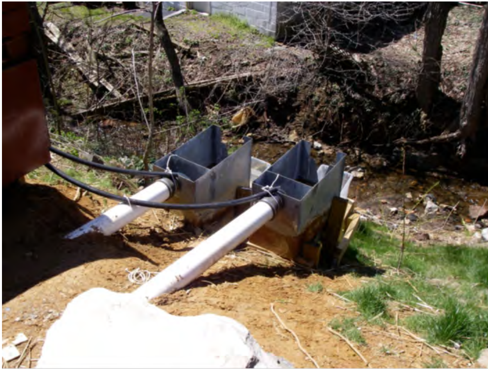
Figure 4-15. Underdrains from permeable pavement equipped with 30° V-notch weir boxes and samplers for flow and water quality monitoring.
