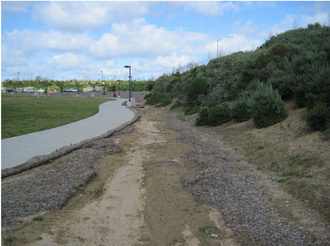
Figure 4-8. Erosion caused by excessive flows in a bioretention swale.
