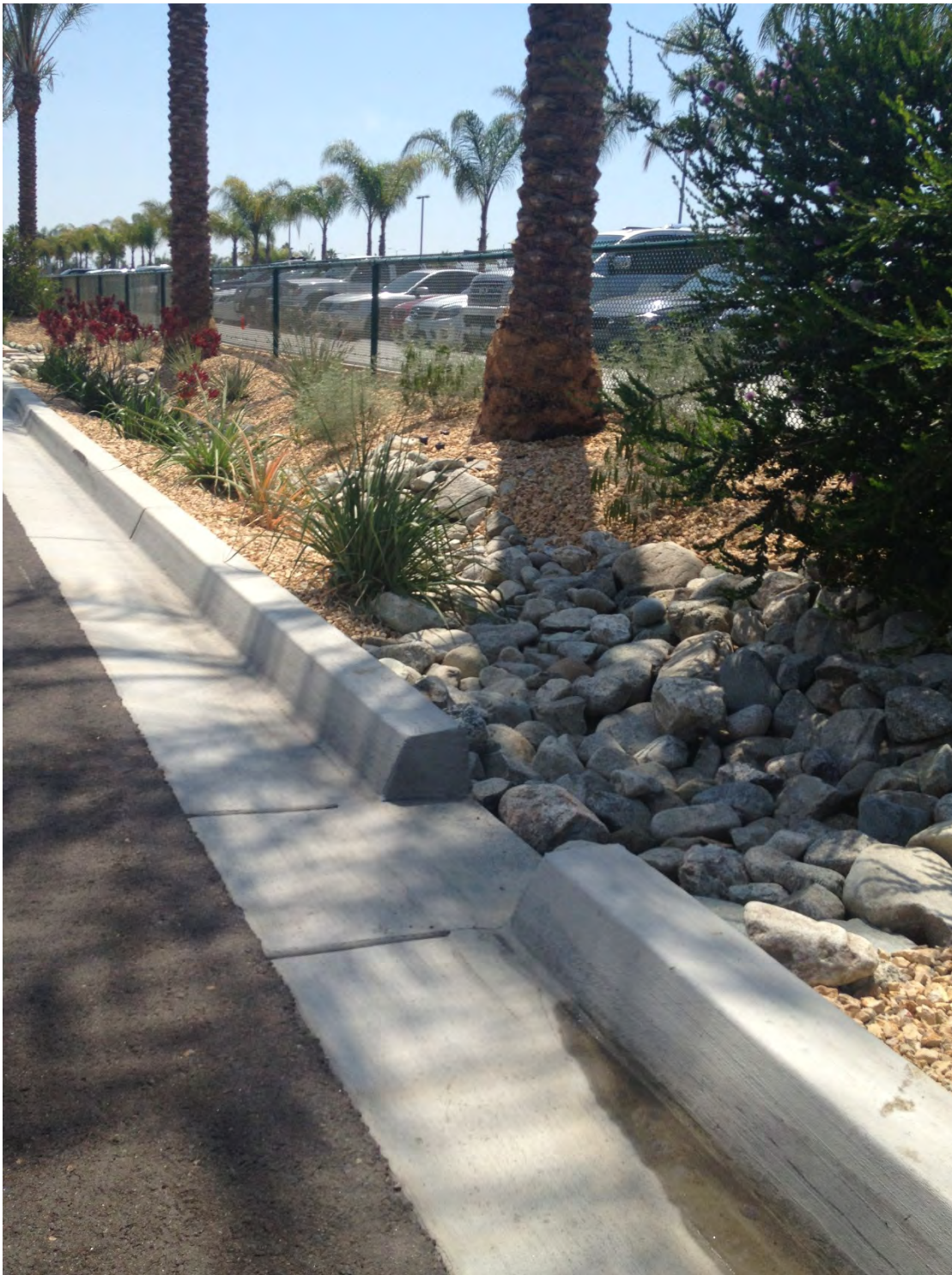
Figure 4-22. Curb cut and cobble energy dissipation at inlet to rock infiltration swale.
