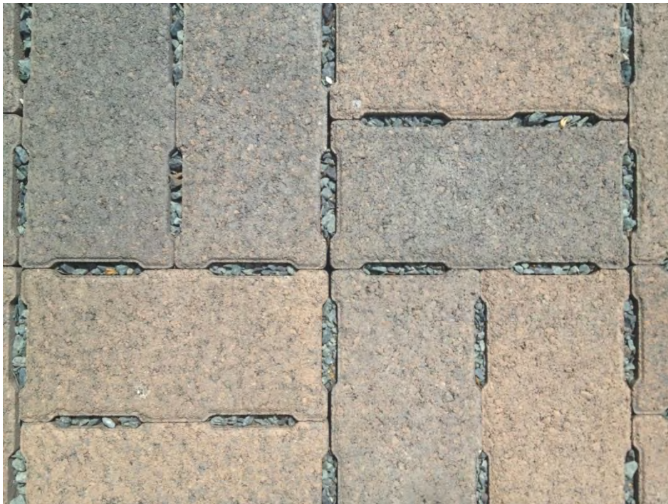
Figure 4-25. PICP was chosen as the surface course for this application. Bedding and joint fill material consists of washed ASTM No. 8.
