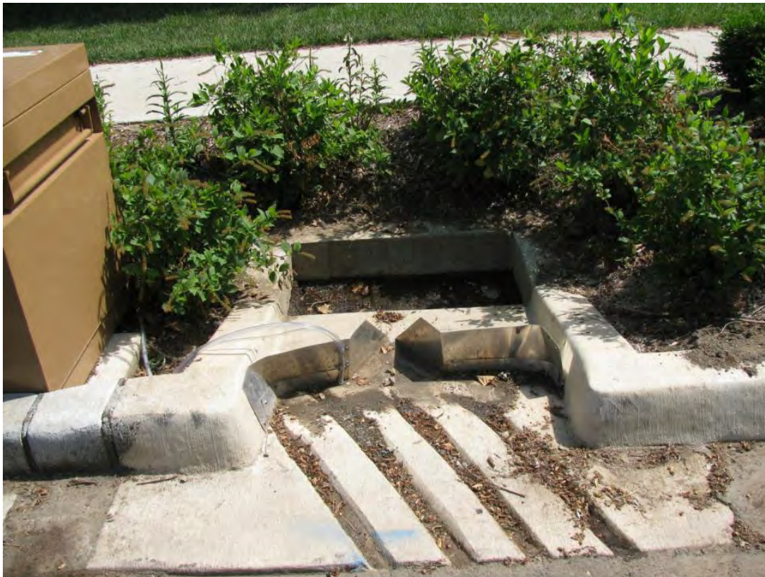
Figure 4-17. Poorly installed H-flume at the inlet to a bioretention area in which the invert of the weir is too low and tailwater from the bioretention will interfere with measurement.
