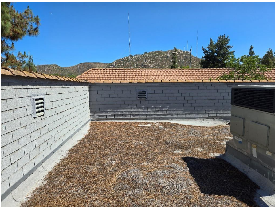
Facing North, looking at 6 th AC unit, North of main roof access door
