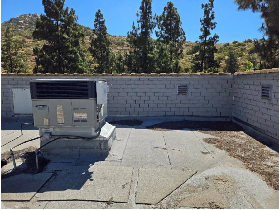
Facing East, looking at 3 rd AC unit, South of main roof access door
