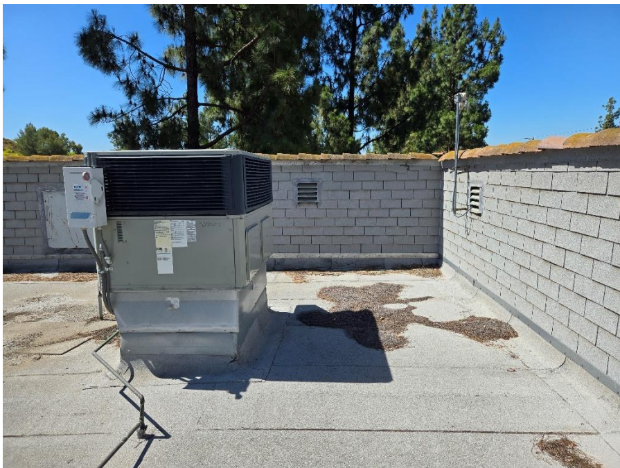
Facing South, looking at 2 nd AC unit, South of main roof access door
