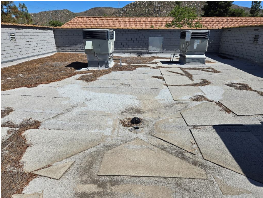
Facing North, looking at roof drain and overflow at middle of roof
