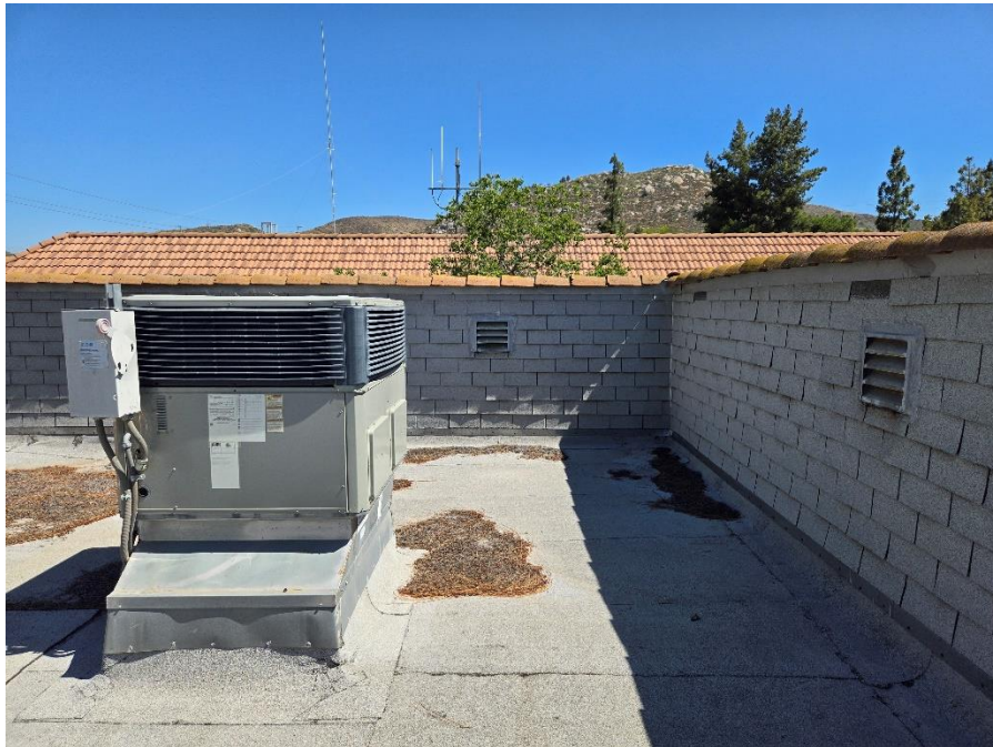
Facing North, looking at 5 th AC unit, North of main roof access door
