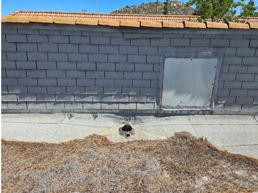
Facing North, looking at roof drain and overflow at North end of roof
