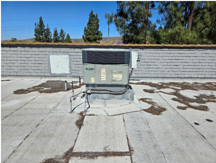
Facing West, looking at 1 st AC unit, South of main roof access door
