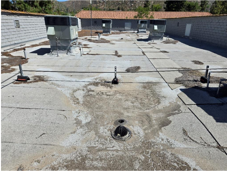
Facing North, looking at roof drain and overflow at South end of roof
