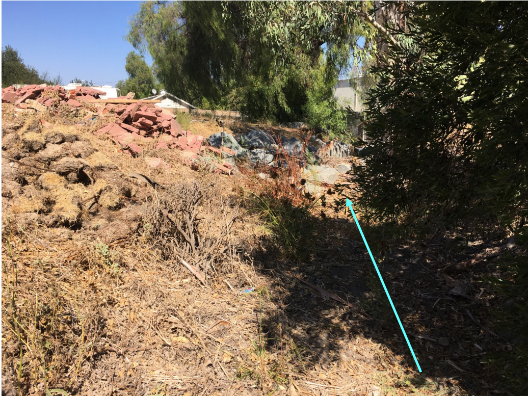
10. Downstream section of drainage channel, with path of flow marked by blue arrow.
