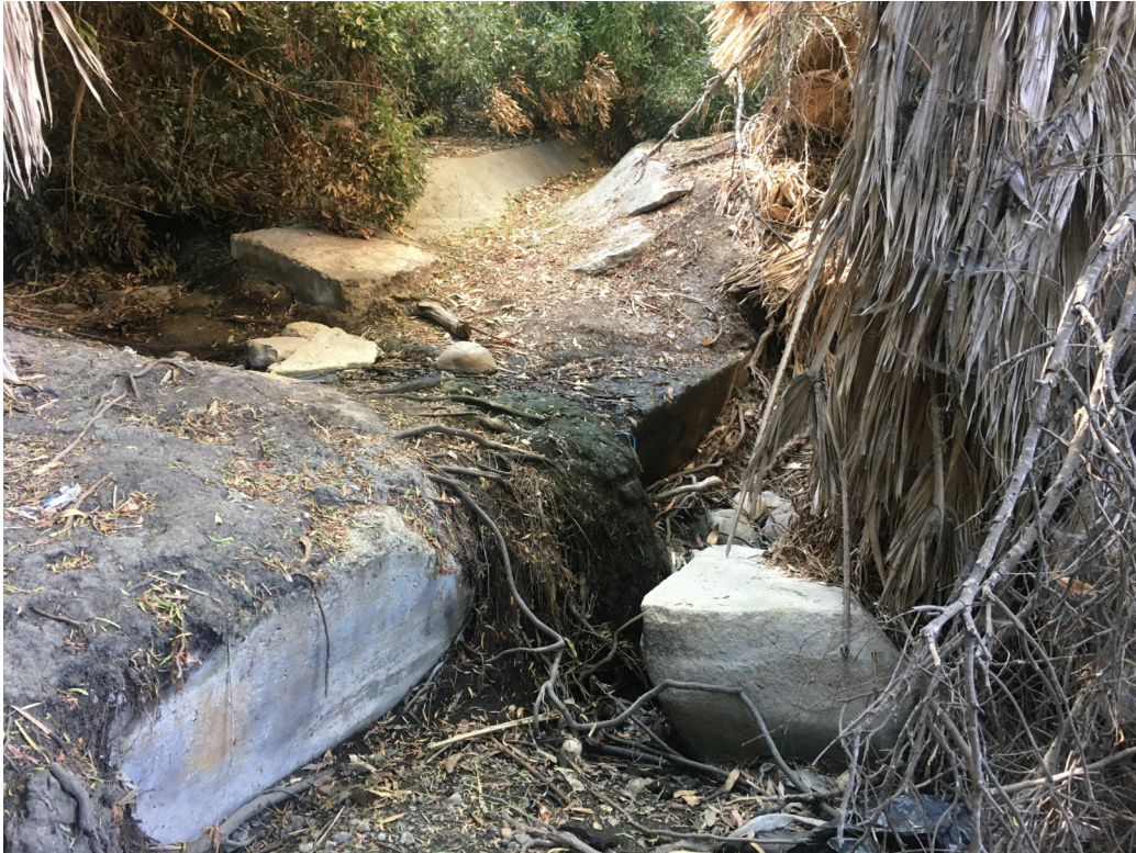
8. Upstream end of drainage where culvert releases water near southern property boundary. Culvert is now hidden under fallen eucalyptus (upper left).
