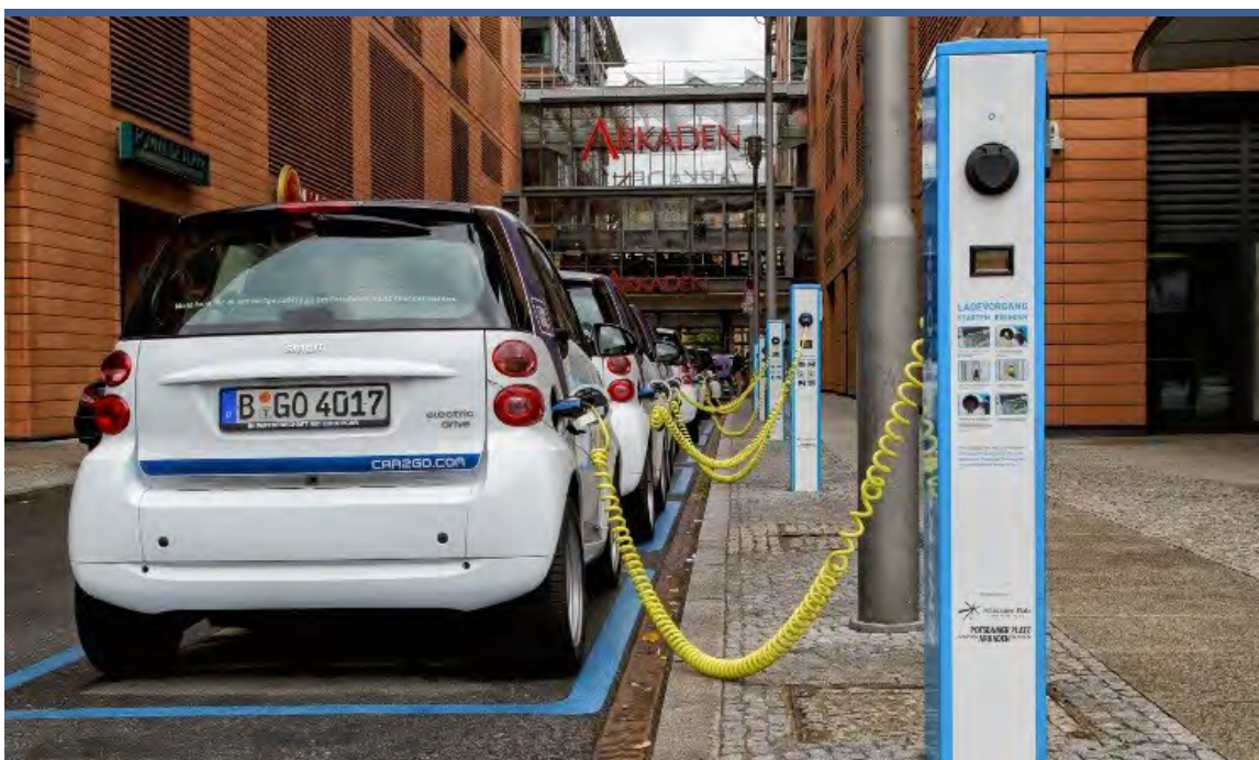
M-3.4: Install E-Vehicle Chargers
